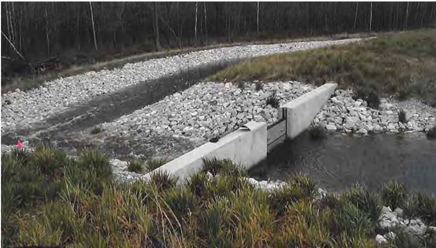
Loop Wetland: System Discharge (Wetland 2 Outlet).
