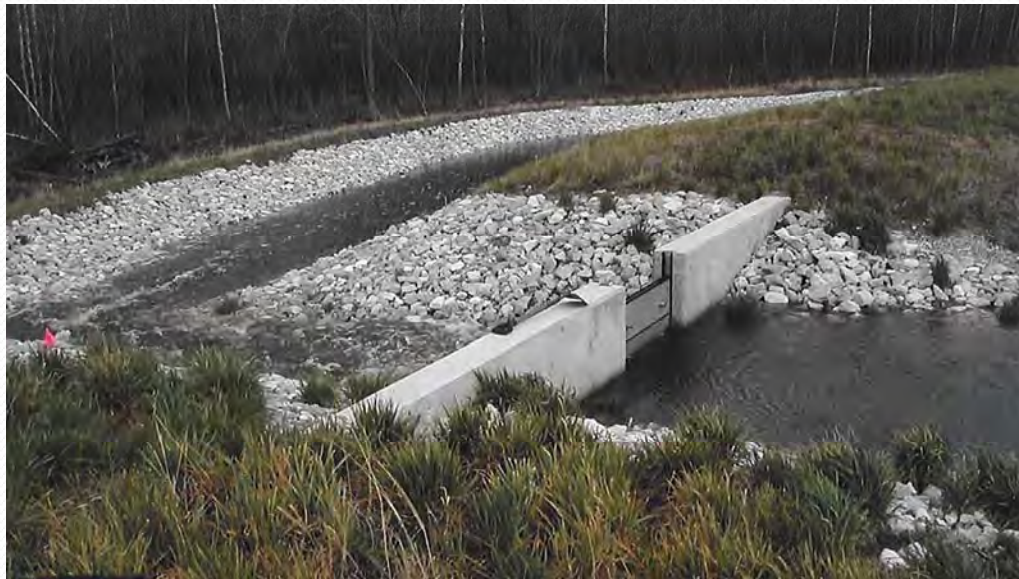
Loop Wetland: System Discharge (Wetland 2 Outlet).
